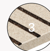
GROOVE WITH EPOXY FILLING
