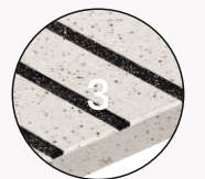
GROOVE WITH EPOXY FILLING
